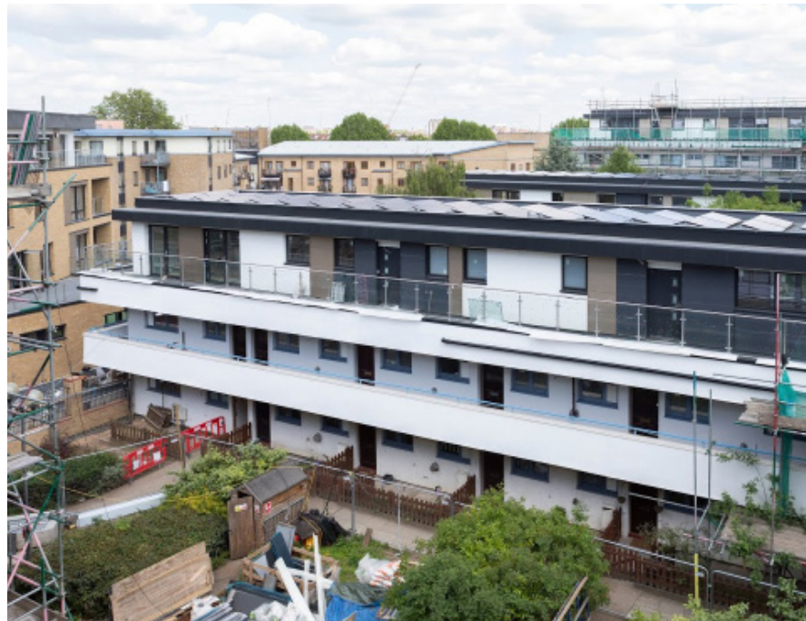
An extra storey on each block in place of the pitched roof
